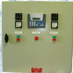
Compressor starter- and control panel
